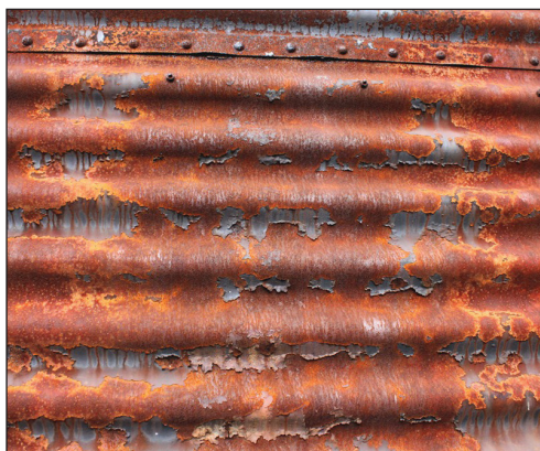
Fig 2.21: Corroded iron sheets due to effects of acidic rain
